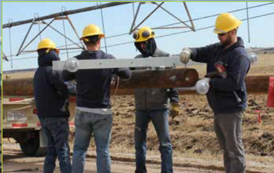
Shayde Linabery, Christopher Stutzman, Kory McManigal, and Will Obrinsky frame a pole.
