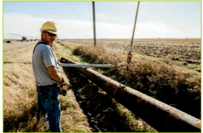
Keith Hoffman works the controller for the digger truck to lift the pole into place.
