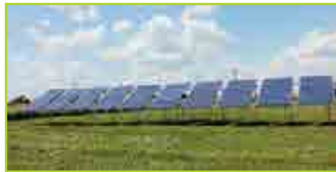
First solar array in Perennial's district.
