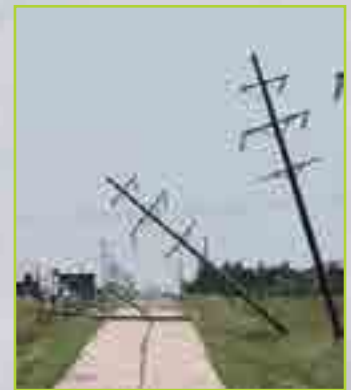
Severe storms damaged lines throughout the district and forced the closure of numerous roads.
